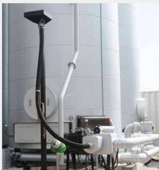
Filling pump with HD8 and manifold with valves.
