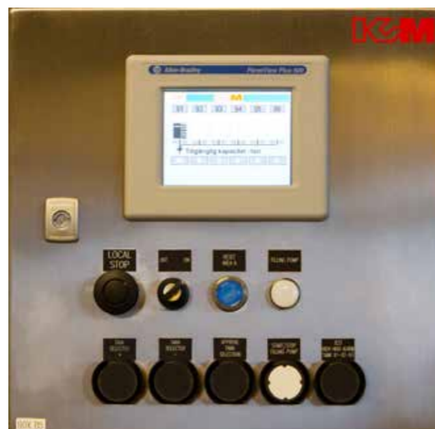
Filling pump control box with HMI display built into a stainless steel cabinet.
